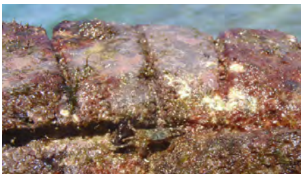
MARINE GROWTH ON SURFACE
